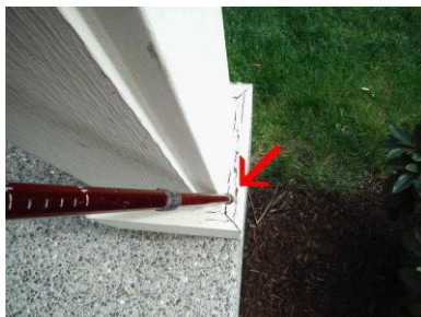
paint/caulk needed front column trim
