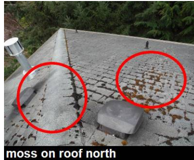
moss on roof north
