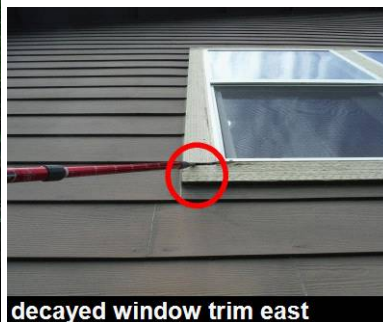
decayed window trim east
